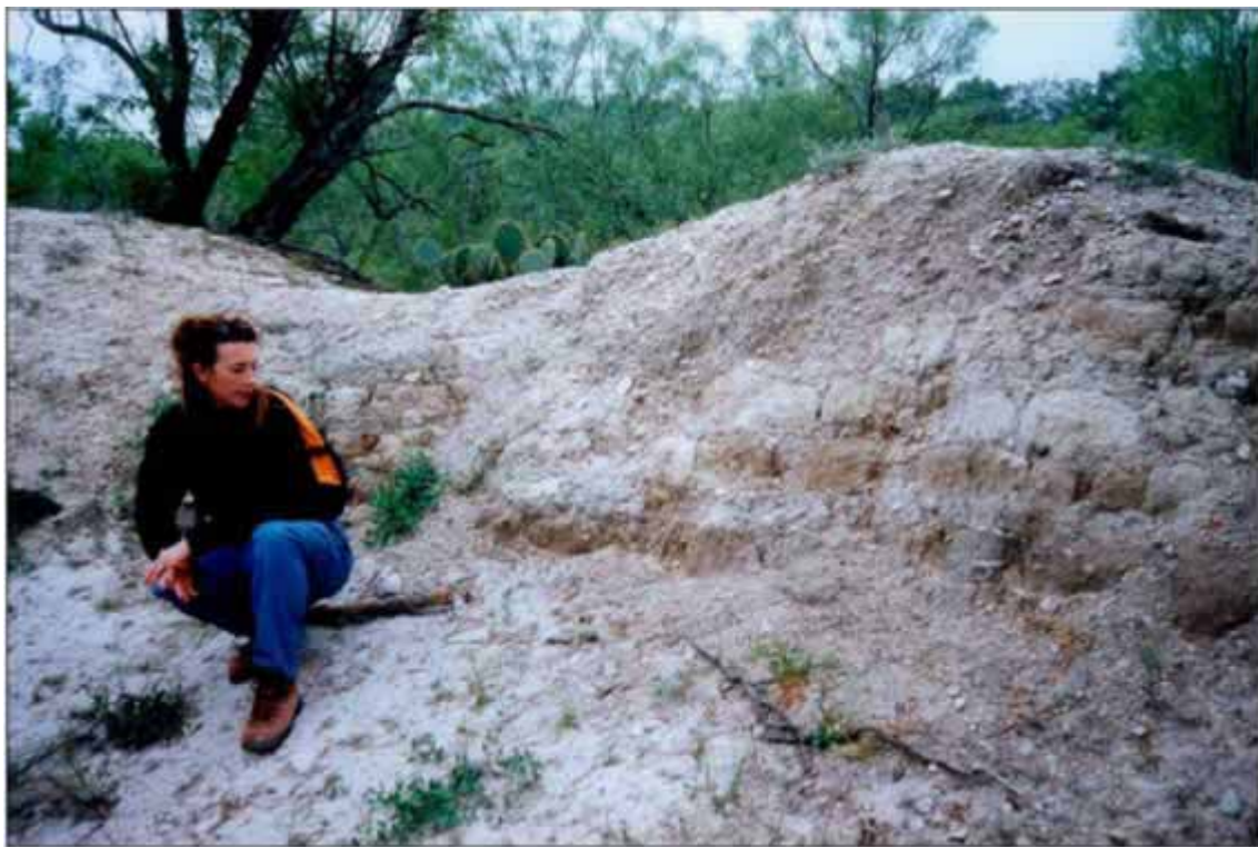
Figure 9. Eroded section of adobe wall.
